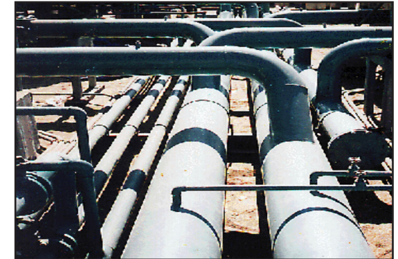
Completed piping system after 10 years
