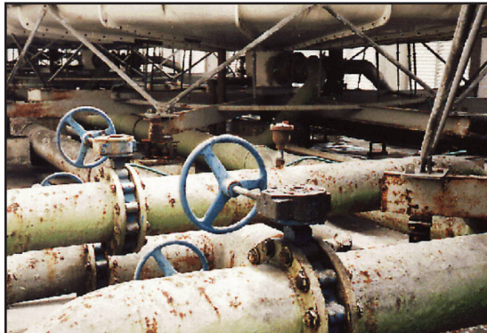
Original piping after 6 months
